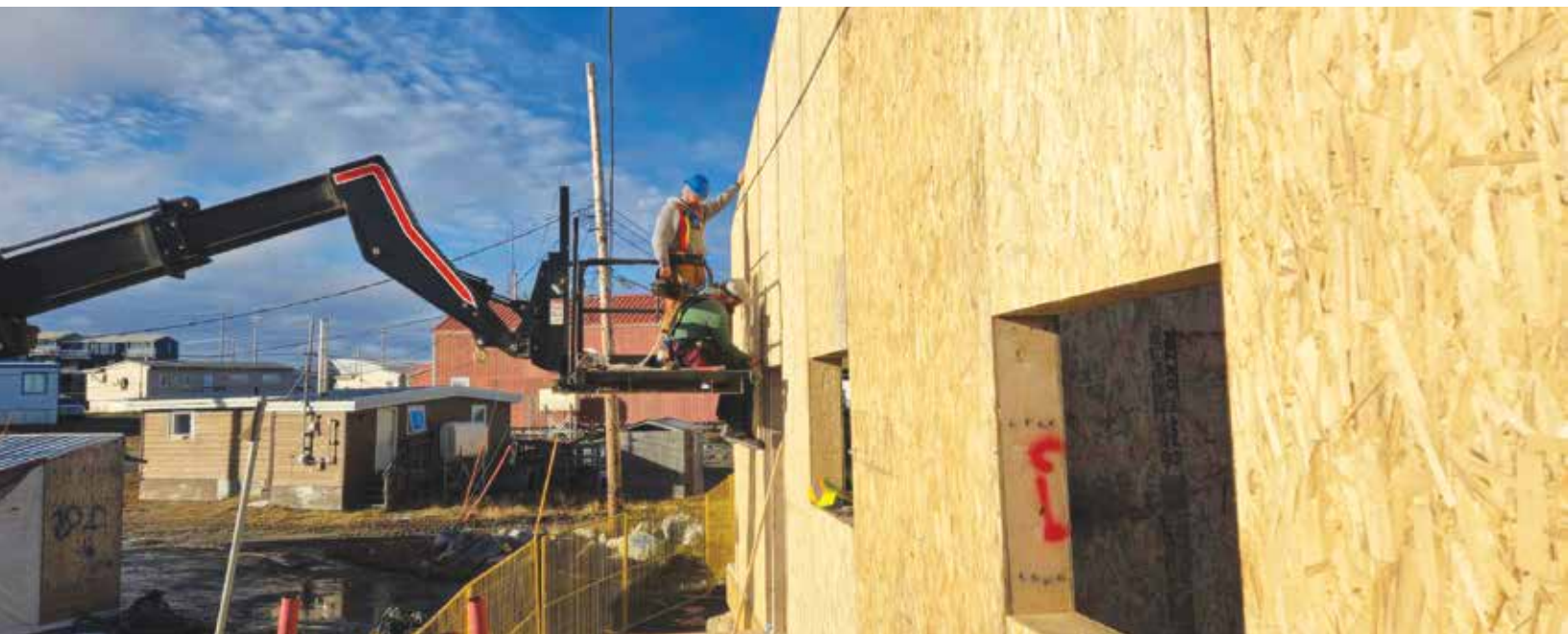
BELOW: Crews install exterior wall panels as part of student-led housing construction.
